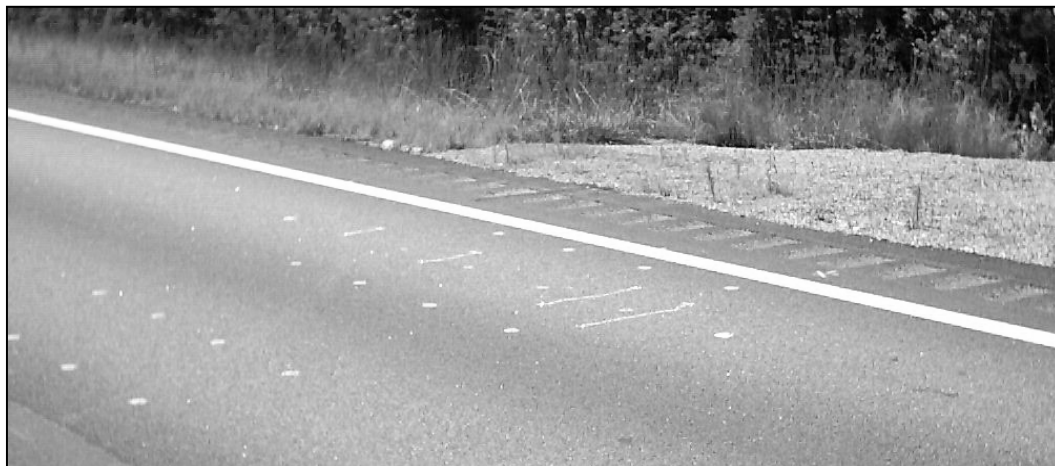
Figure 4.38 Transverse Cracking in the Wheelpath - Section N8.
